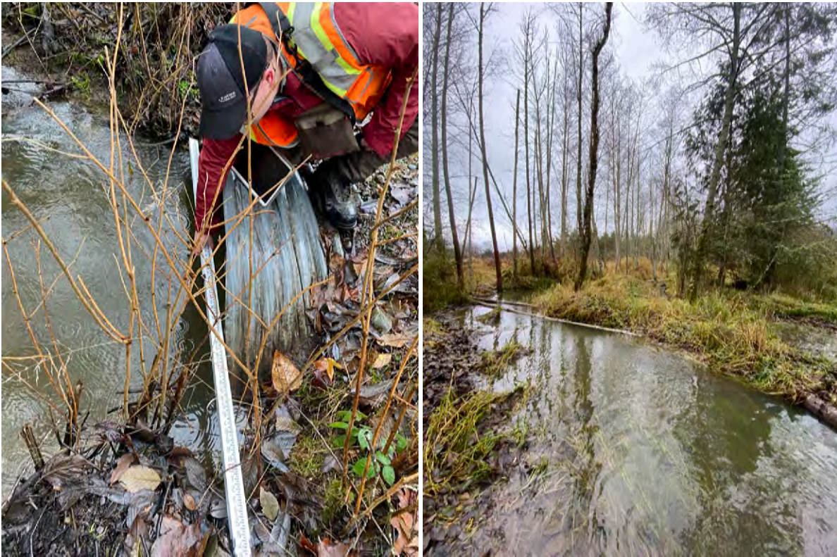
Wrucha Private Road Culvert and Combined Colony/Harrison Creek Flow Just Downstream
