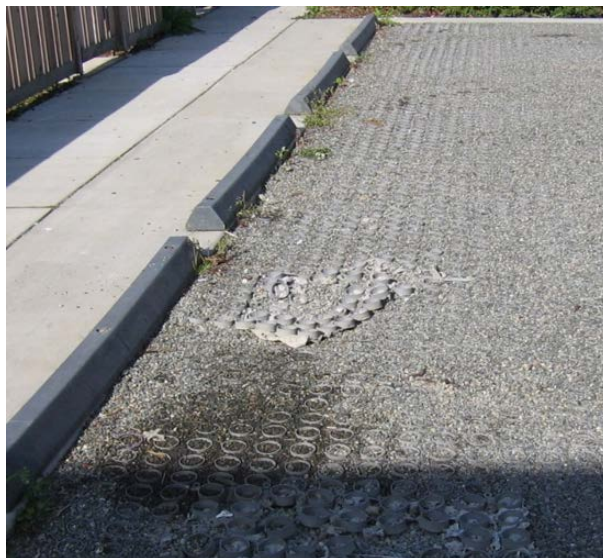
Improperly installed open celled plastic grid
