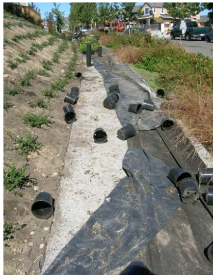
Poorly maintained TESC during construction (note the upslope soil posing a clogging concern for the underlying pervious concrete sidewalk)
