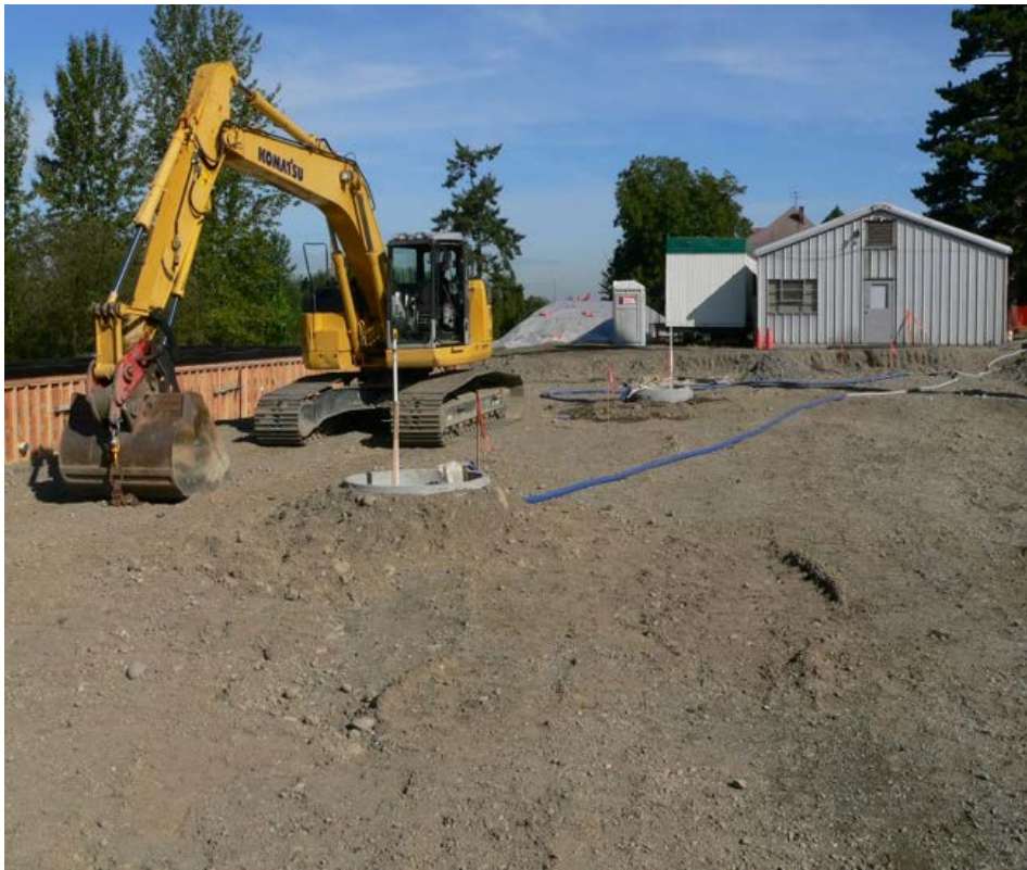
Example of an excavator pulling material back to ensure subgrade is at the proper final elevation without allowing heavy equipment on the finished subgrade
