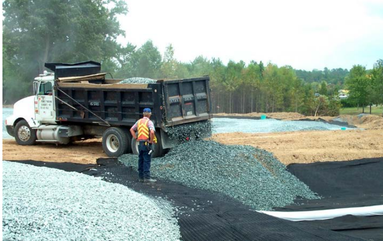
Example of aggregate base being loaded around the edges of a facility in order to protect the subgrade
