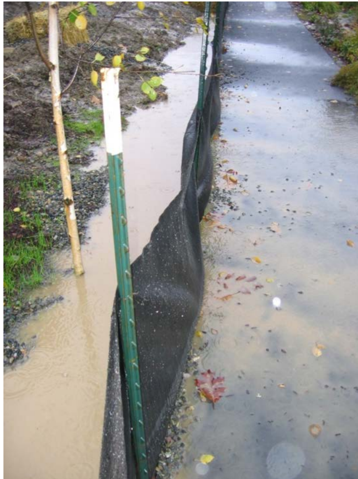
Example of a situation where TESC is in place and functioning properly, but additional protections need to take place due to extraordinary climactic conditions
