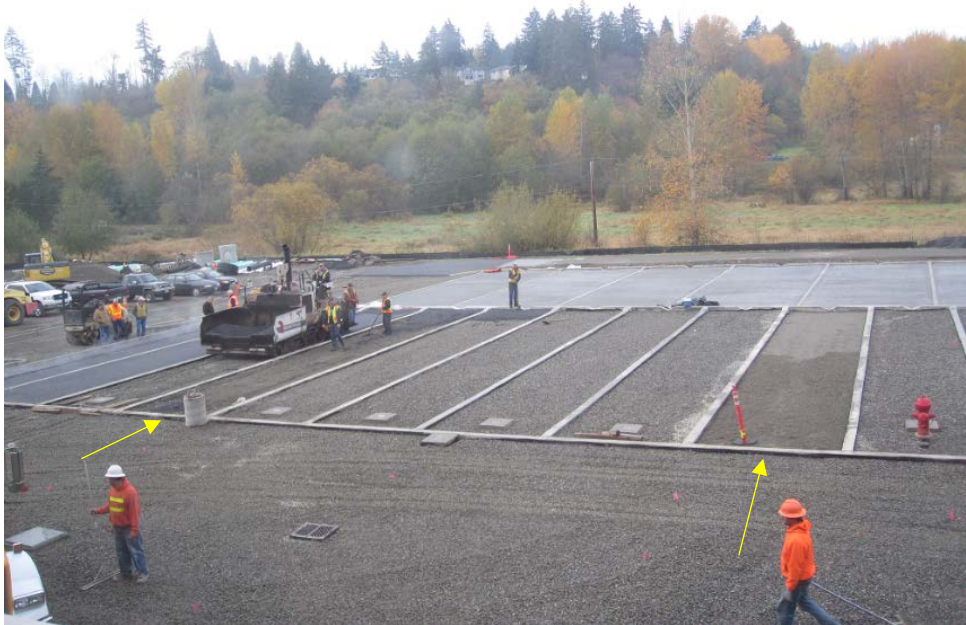
Installation of a permeable asphalt study area at Washington State University in Puyallup. The cells denoted with yellow arrows were installed as traditional, impermeable asphalt. The rest of the cells and the lot in the foreground were all installed with permeable pavement with choker course visible (Note the choker course has visibly larger graded material (for infiltration) than the traditional asphalt foundation.)
