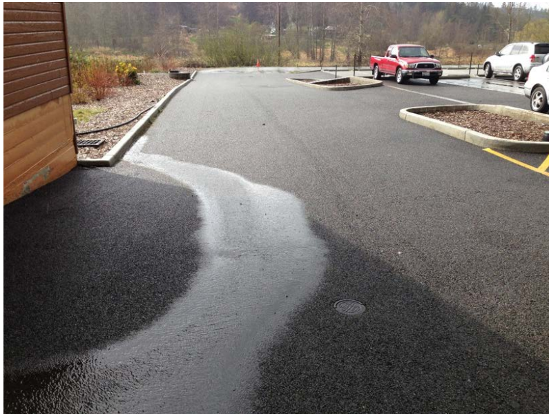
An example of runoff from an impervious pavement. The transition sloped from impervious pavement toward porous asphalt, causing sediment to clog the system in the flow pattern
